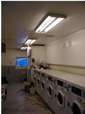
Washeteria lobby with T8 upgrades.
