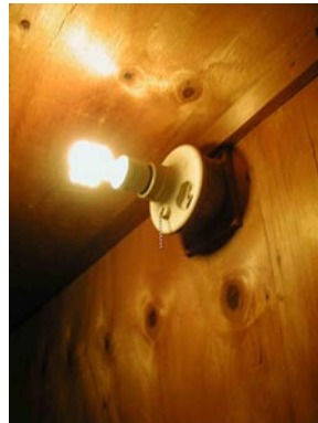
CFL installed in Washeteria sauna.
