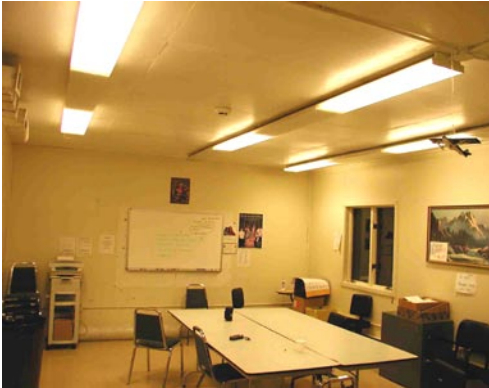
IRA Boardroom upgraded with T8s and fixtures taken offline.
