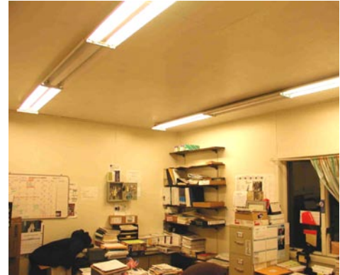
IRA Administrator Office upgraded with T8s.
