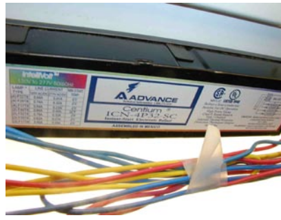
Electronic ballast installed.
