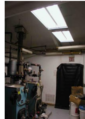
Washeteria boiler room with T8s
