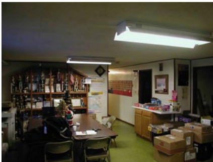
City office meeting room with T8 upgrades.
