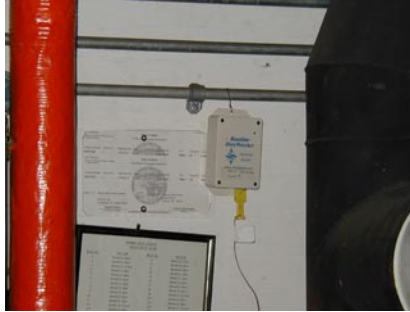
Run-time data logger on existing Golovin water plant boiler
