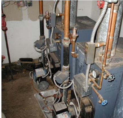
Existing Boilers - Goloviin Duplex Teacher Housing Building
