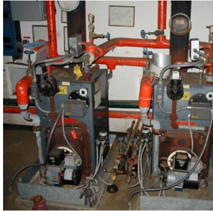
Existing BSSD Water Treatment Plant Boilers
